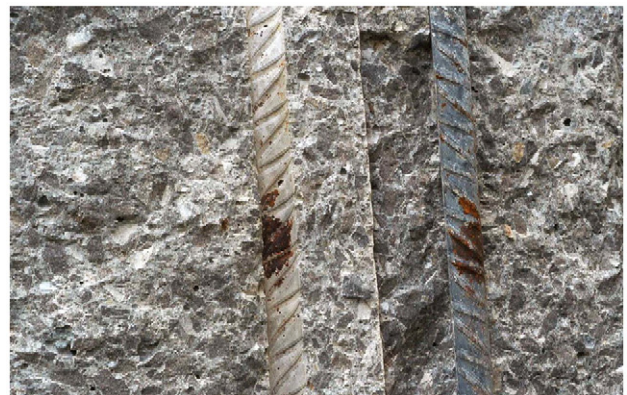
Fig. 5. Corrosion of carbon steel embedded in C35/45 concrete slabs without chlorides and partially immersed in 3.5% NaCl solution at the end of the tests.
